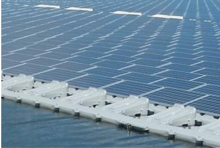
Photo of a similar floating solar installation
